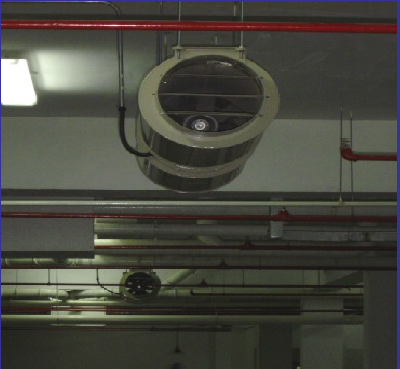
Jet Fan Front View (Installed)
