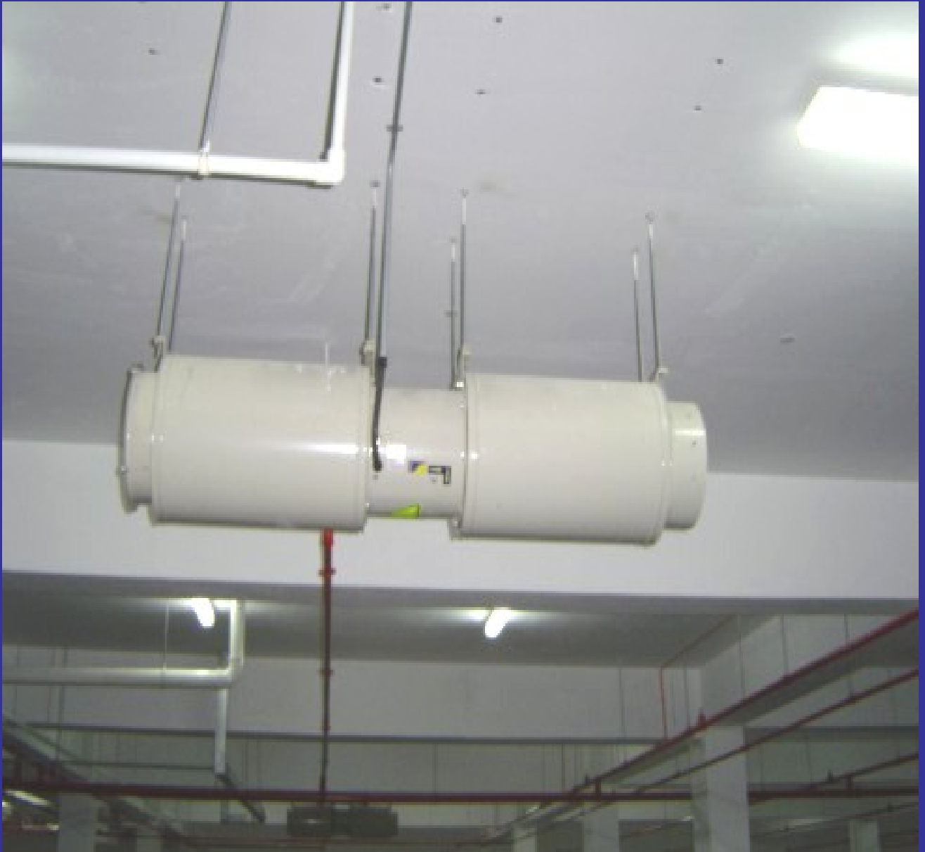
Jet Fan Lateral View (Installed)
